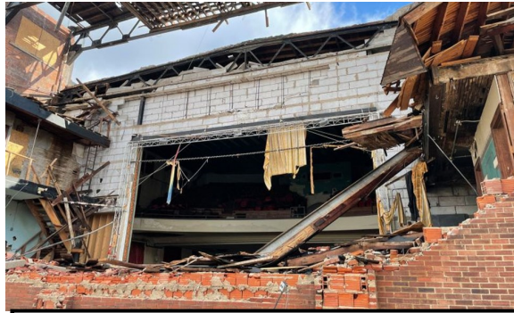
The back of the heavily damaged American Legion Post 26 building in downtown Mayfield, Ky., where a large theater screen used to be. (Photo by Henry Howard.)
