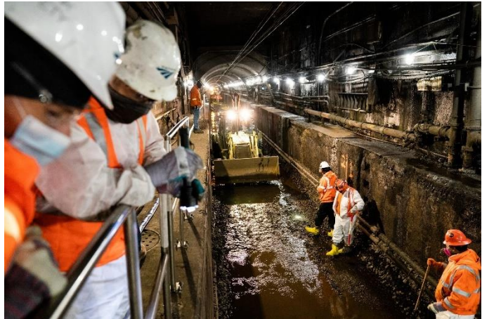
Amtrak workers repairing a partially flooded train track bed in Weehawken, N.J.
